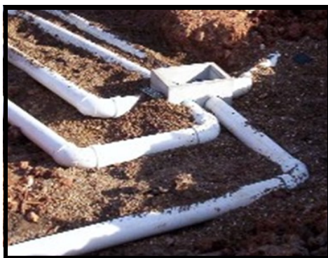
Concrete distribution box
