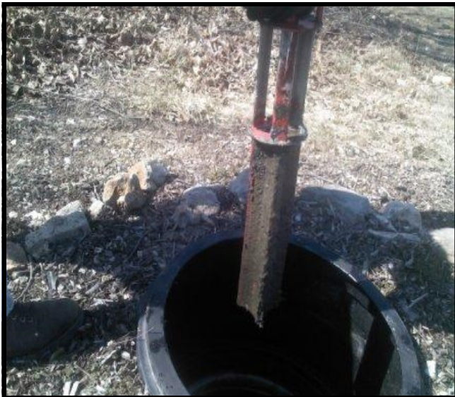
A dirty EFFLUENT screen. This screen is located in the outlet baffle of a septic tank.
