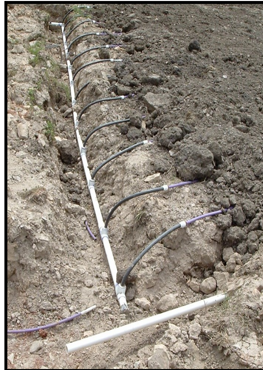
Subsurface Drip Dispersal. A manifold trench and supply manifold line is shown with flexible pipe connected to the small diameter drip irrigation lines. The return manifold from the opposite end of the zone is shown in the foreground. Drip lines are often plowed into the soil; this photo shows suitable imported soil used to cover the drip lines.
