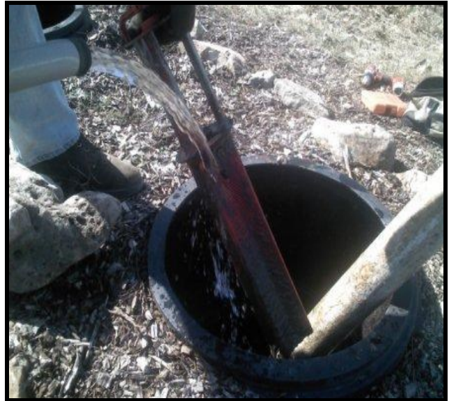
Properly cleaning a dirty EFFLUENT screen.
