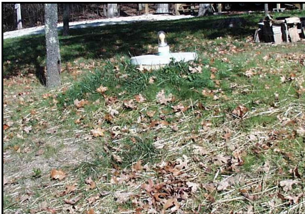
MALFUNCTIONING Holding Tank. The bright, lush green grass around the top of the manhole cover is evidence that the HOLDING TANK has been leaking due to the lack of proper MAINTENANCE and routine pumping.
