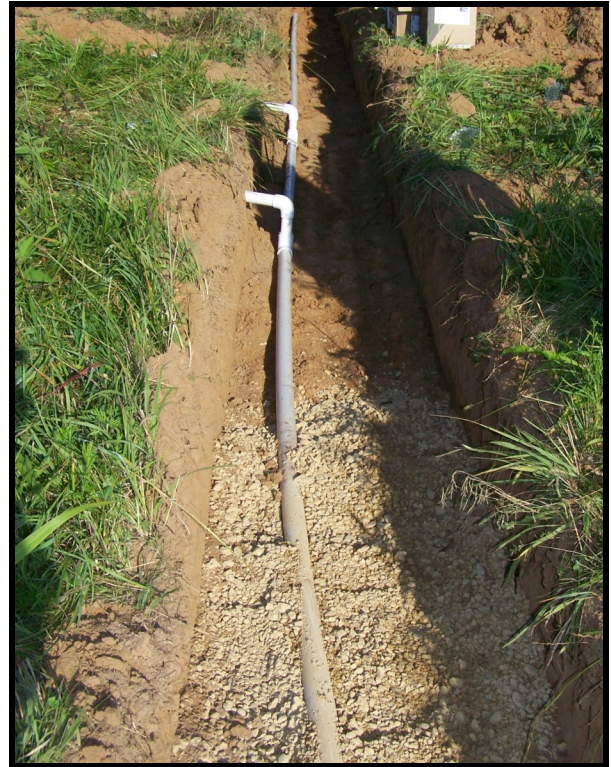
Low Pressure Pipe Manifold. The manifold trench and connections to LPP valves and distribution lines.
